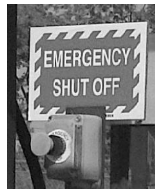
Figure 13. Emergency shut-off buttons for compressed natural gas maintenance facilities and fueling infrastructure
