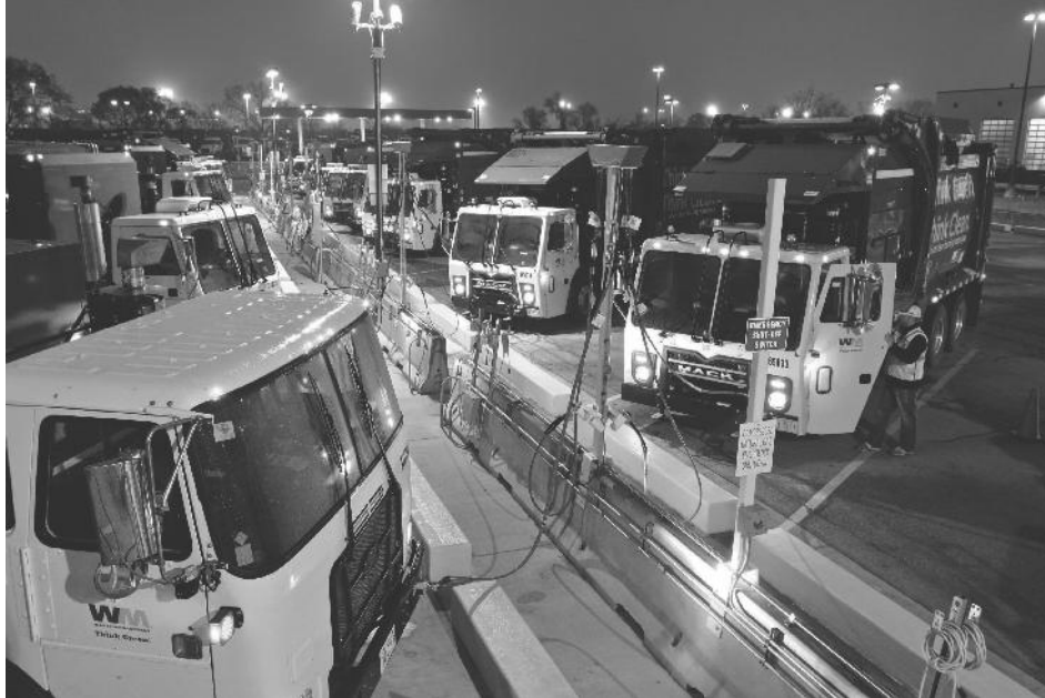
Figure 24. Waste Management time-fill compressed natural gas station in Chicago
