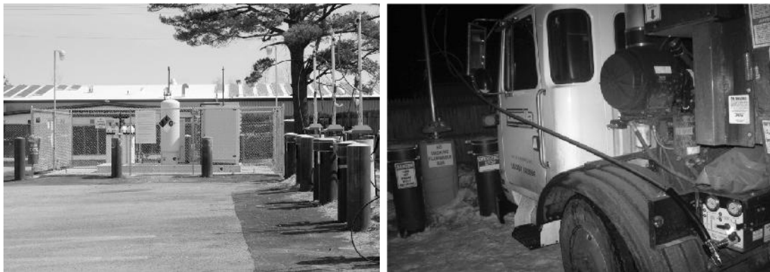
Figure 22. Casella Waste Systems time-fill compressed natural gas station for refuse vehicles
